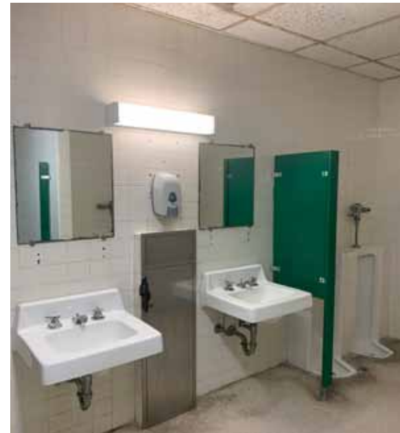
Restrooms are dated, not ADA compliant
